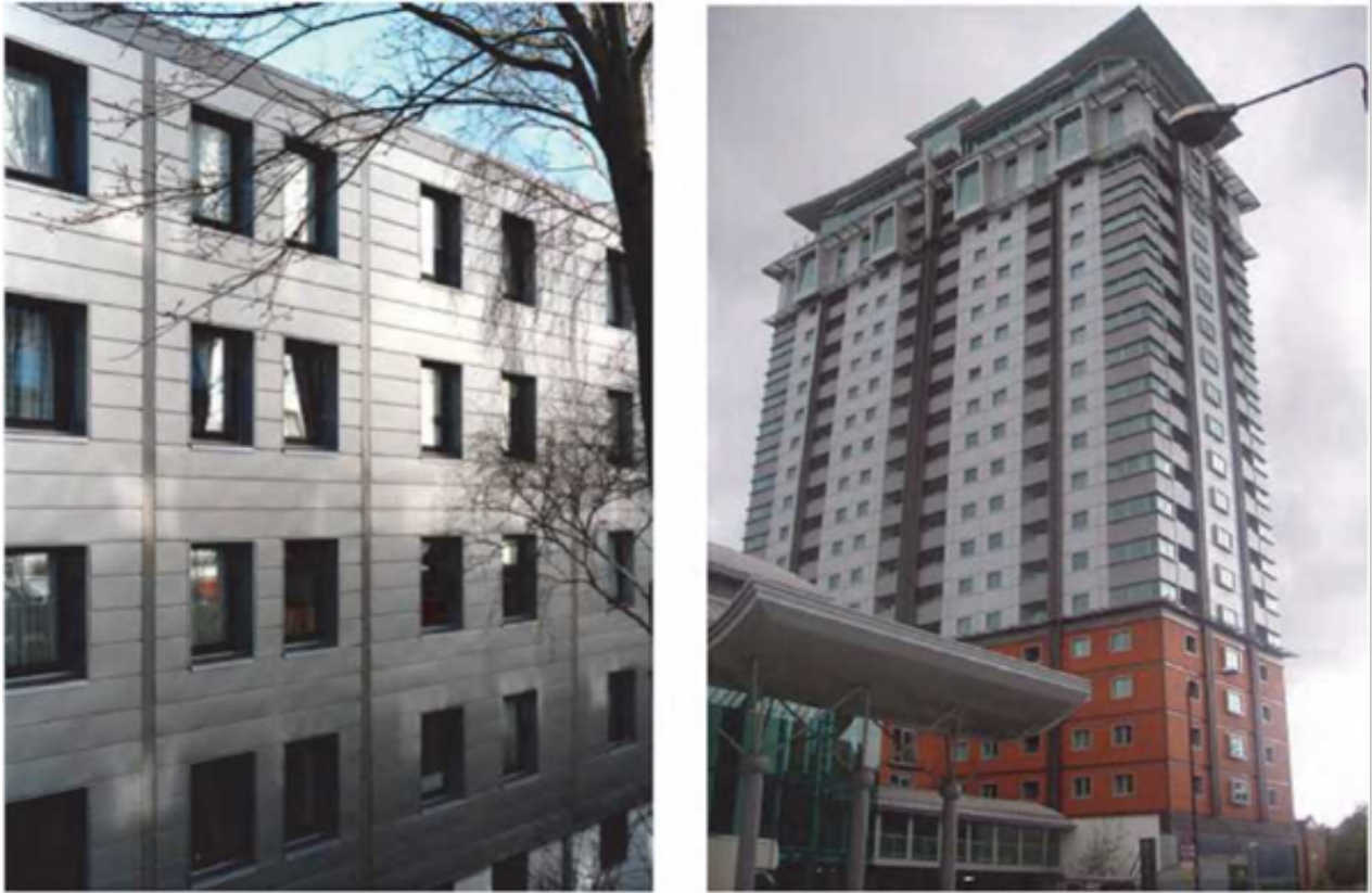
Figure 1. Examples of installing new facade systems on old facades of buildings with concrete wall panels. The new facade systems consist of horizontal metal panels
