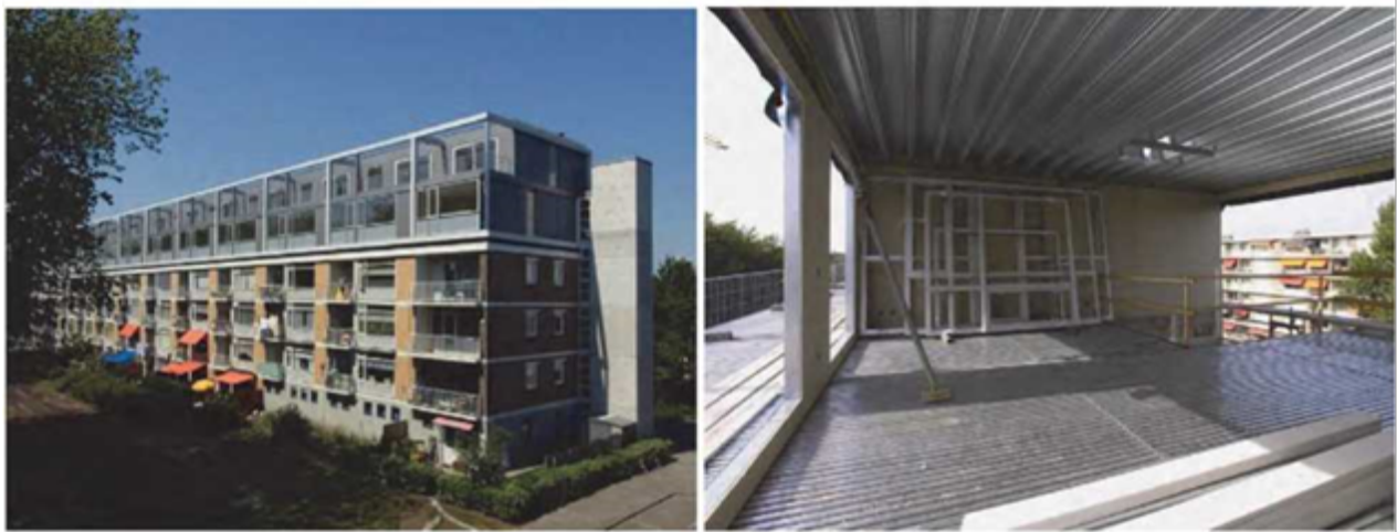
Figure 2. Two-storey superstructure made of light steel frame on an existing building, Rotterdam
